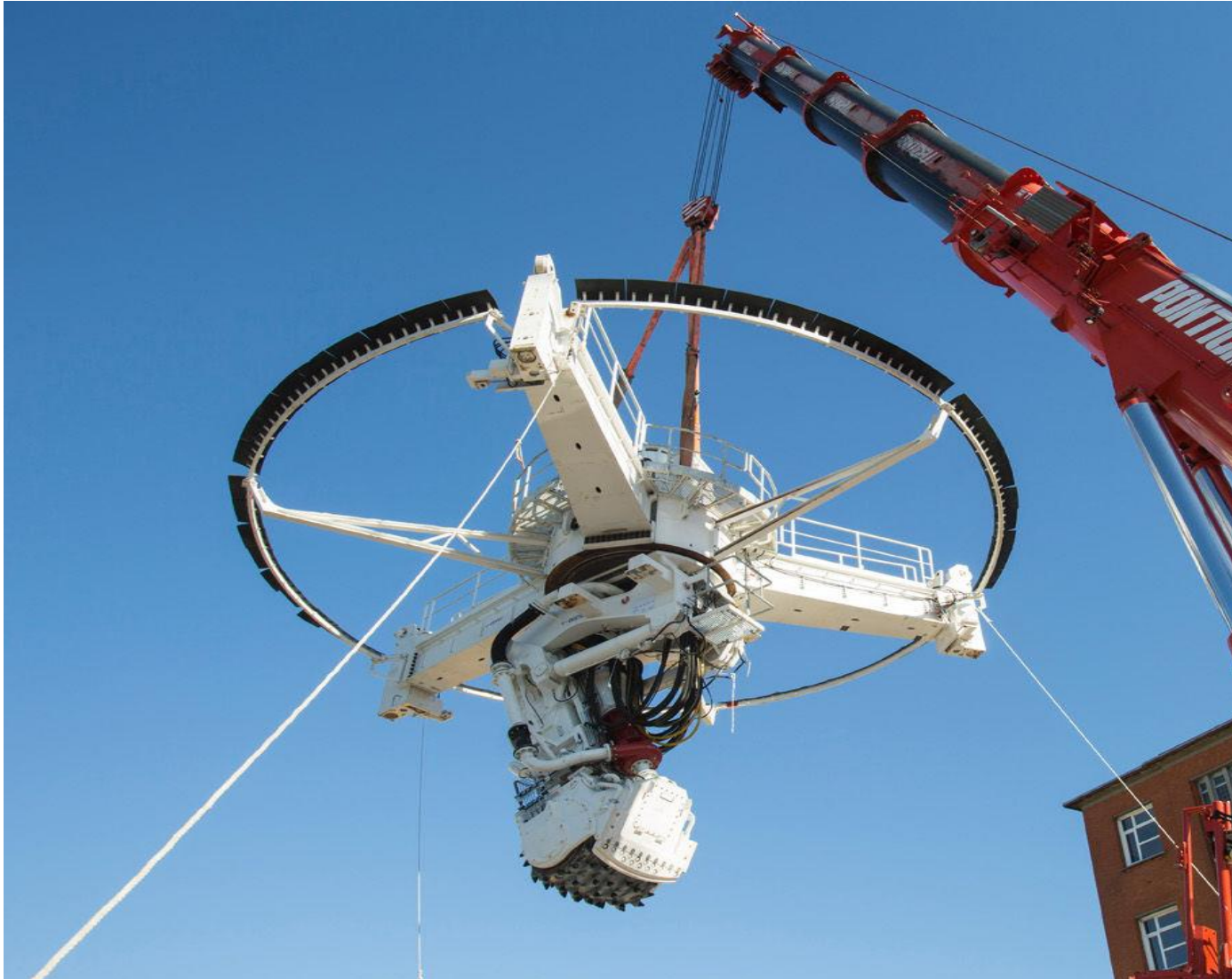
Vertical tunnelling on section T3C of Line 15 South of the Grand Paris Express
